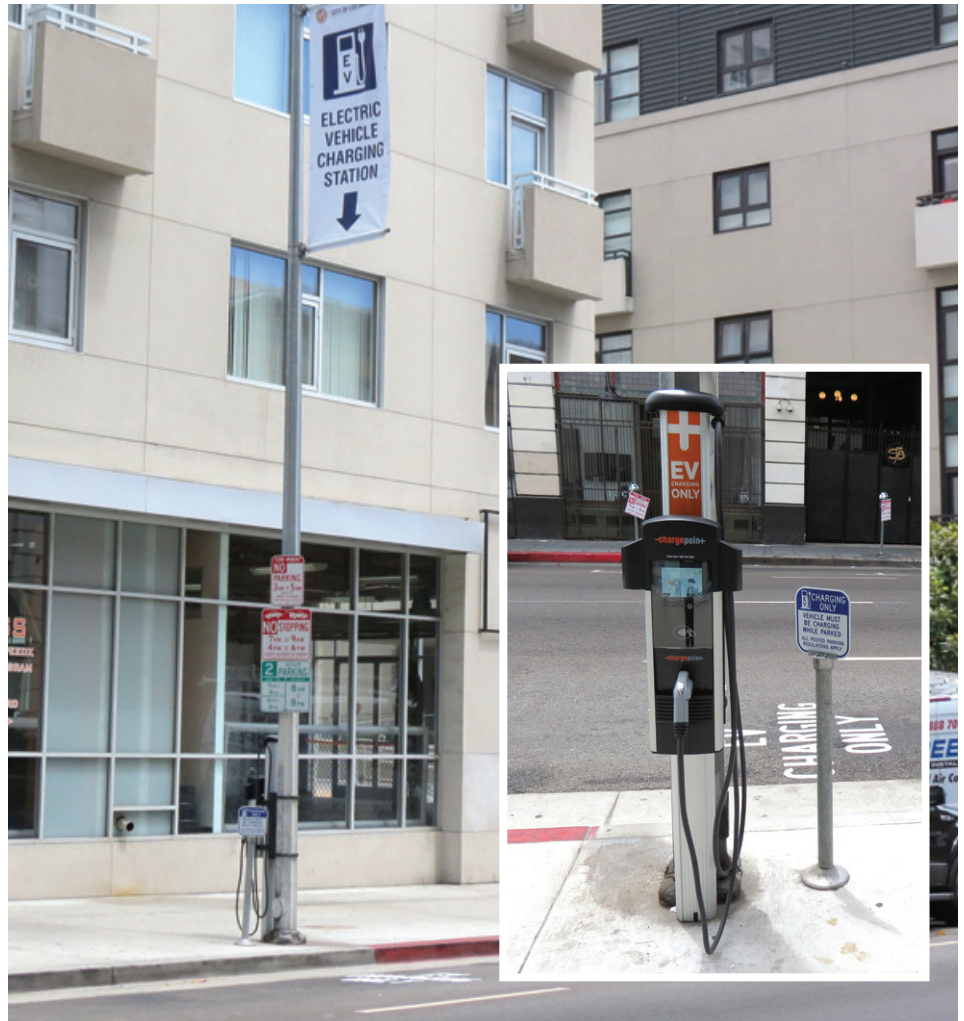
EV drivers can charge their cars on 4th Street. Banner sign shows drivers location. (Inset photo) Close up of EV charging station
